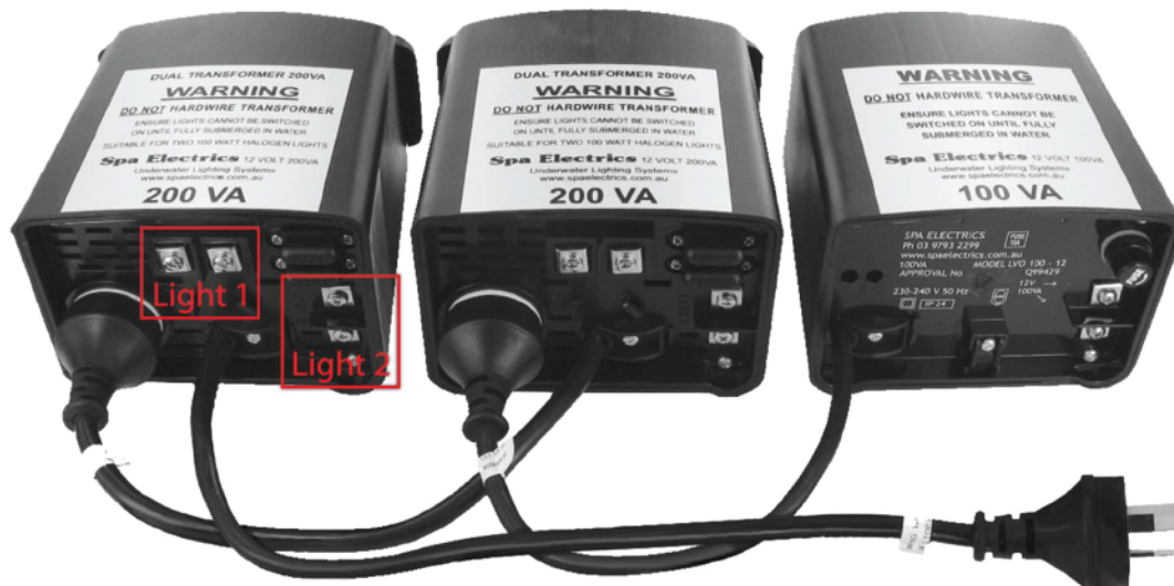
Example of a 5 Halogen light transformer setup.
